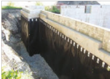
A gap around the basement wall in a home that is under construction.
