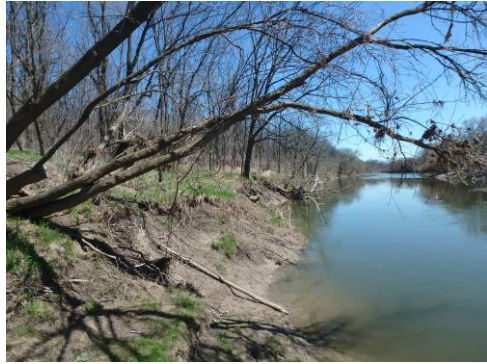
Evidence of toe erosion, including bare banks and fallen trees, April 2016
