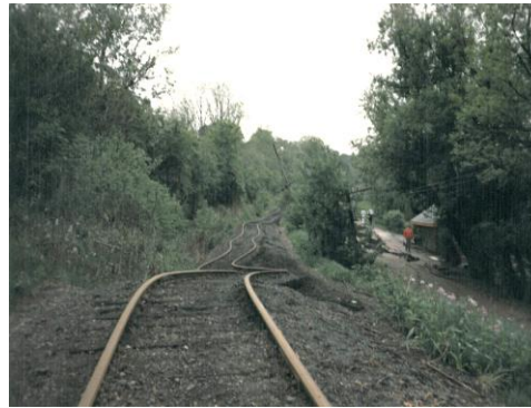
Railway along Beach Road after 1986 landslide
