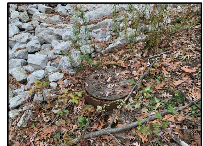
D. Emergency Bank Stabilization Measures to Protect At-Risk Manhole 11
