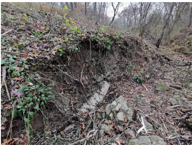
Figure 2-1: Exposed Sanitary Sewer Due to Channel Erosion (Pre-Repair, 2019)
