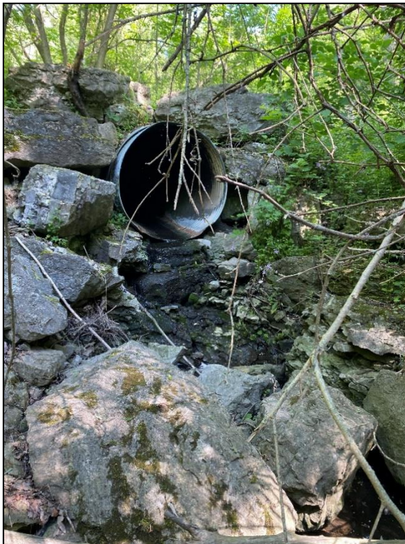
Figure 3-14: Perched CSP Culvert.
