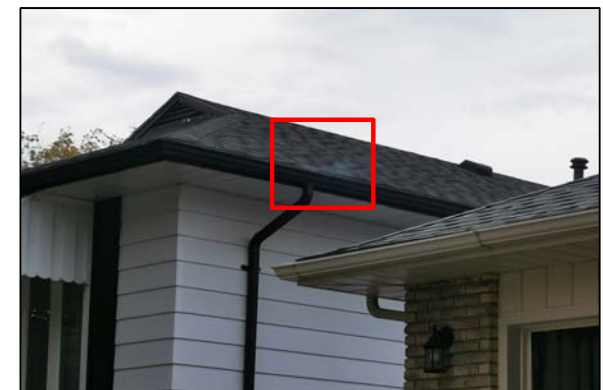
Connected downspout was smoking during the test.
