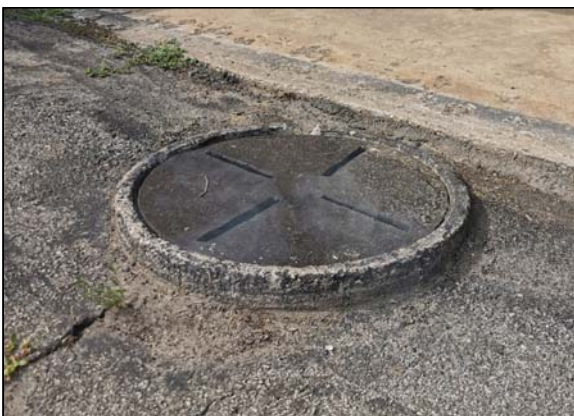
Weak smoking garage catchbasin, indicating potential blockage in storm drain.
