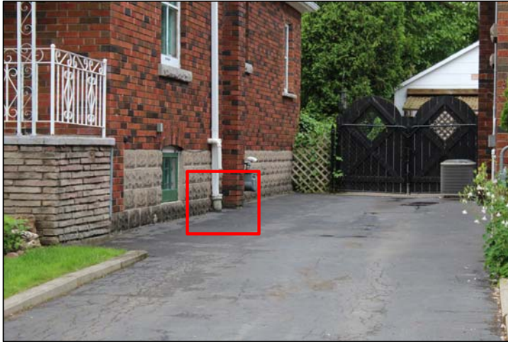
Connected downspouts (eavestroughs) direct flows into the underground sewer system and increase the potential of overwhelming the sewer system during heavy rainfall events.
