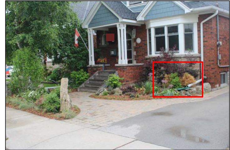
Disconnected downspouts (eavestroughs) direct flows to garden or lawn, which helps promote infiltration, reduce the amount of water entering the sewer system, and delays the time of water entering the sewer system.
