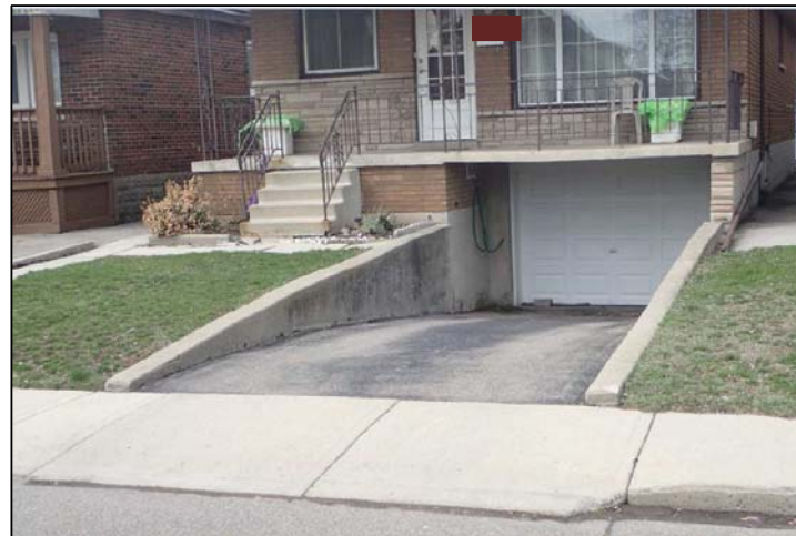
Homes with reverse slope driveways, without trench drainage in front of the garage, could be susceptible to overland flooding.
