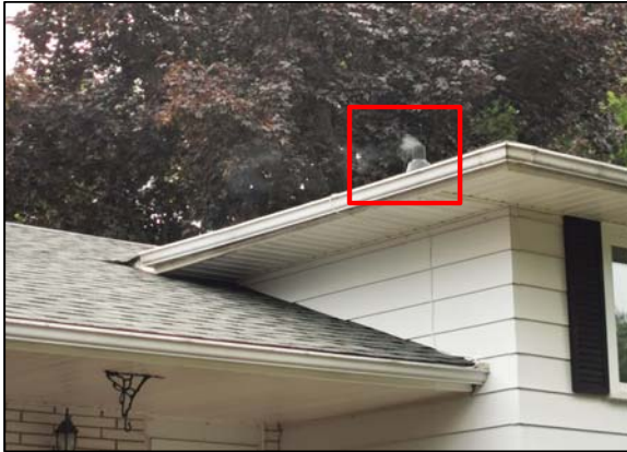
Smoke from plumbing vent, indicating potential cross-connection between sanitary lateral and storm sewer.
