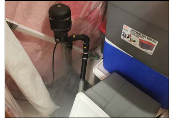
Basement sump pump was smoking, indicating direct connection to storm sewers on street.
