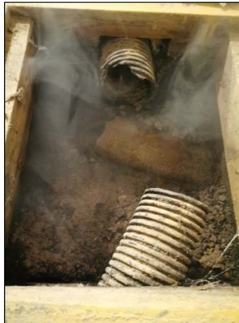
Foundation drain was smoking during the test.
