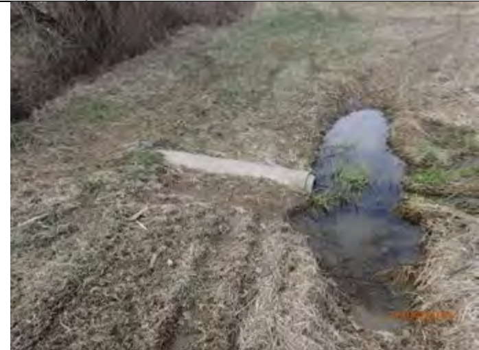
CAPTION: Feature at downstream limit of accessible properties; culvert through fence line. Site visit #1 – April 2018
