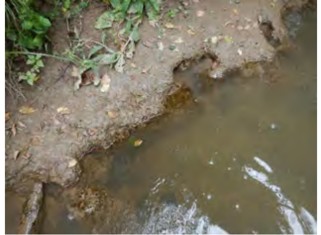
Photo 2: Erosion of clay at bank toe
