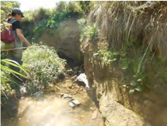
Photo 1: Till/clay banks; bank scour and cantilever failures of bank materials; root exposure
