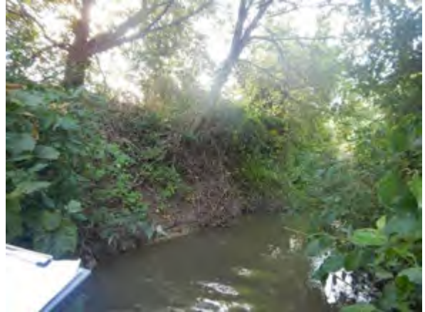
Photo 2: Bank erosion; exposed roots
