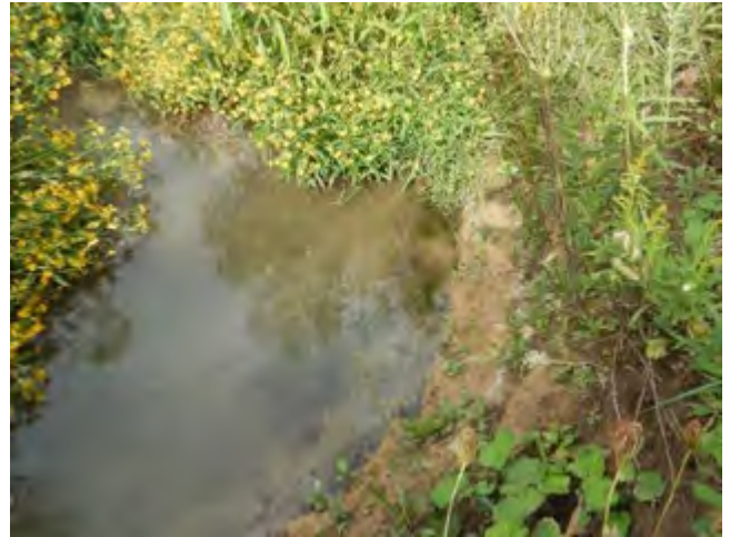
Photo 2: Bank toe erosion into firm till layer
