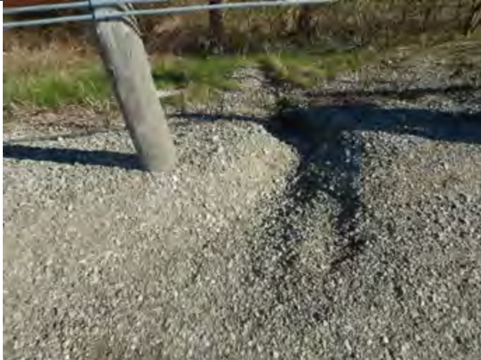
CAPTION: Rill erosion at upstream limit of feature at Powerline Road. Site visit #1 – April 2018
