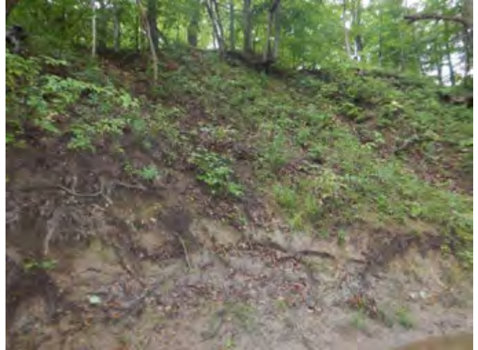
Photo 2: Bank toe scour at valley wall contact
