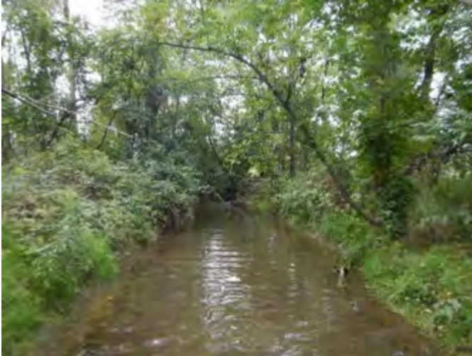
Photo 1: Bank scour, exposed roots, leaning trees
