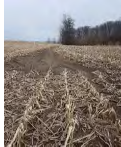
CAPTION: Drainage feature loses definition; downstream view.
