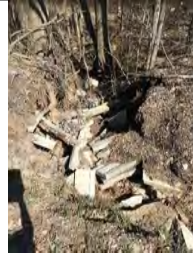
CAPTION: Erosion and concrete slab protection at downstream limit of feature into wooded area. Site visit #1 – April 2018
