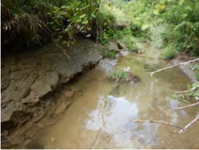
Photo 1: Exposed native till with sand and fine gravel deposits; till eroding at bank toe into blocks / pieces
