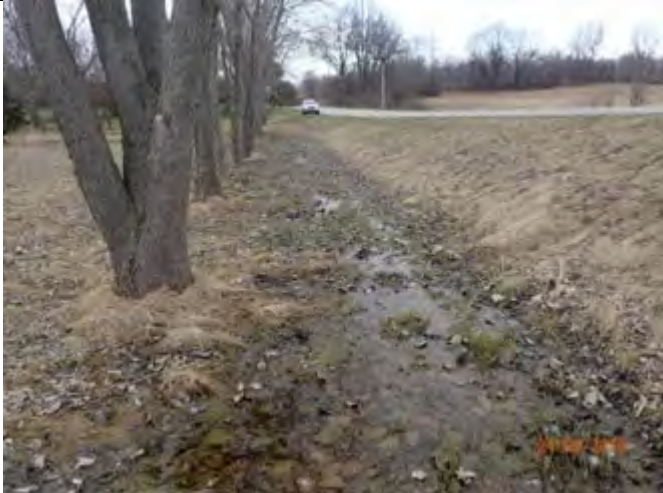
CAPTION: Roadside drainage feature along Golf Road, downstream view. Site visit #1 – April 2018
