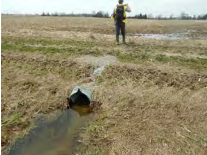
CAPTION: Upstream view of feature through private culvert crossing. Site visit #1 – April 2018
