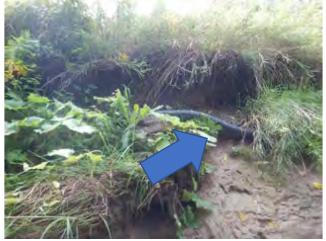
Photo 2: Influences from residential land use: drainage, water taking, urban debris
