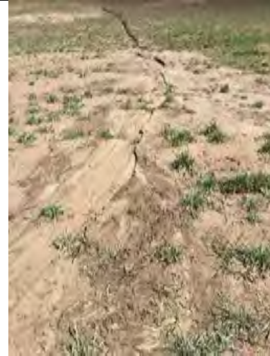
CAPTION: Depositional nature of rill feature at downstream limit. Site visit #1 – April 2018
